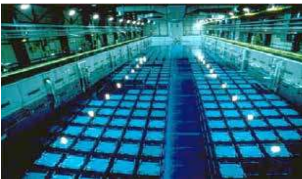
Figure 1 – Main spent fuel pool in La Hague
